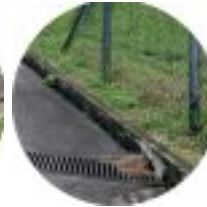
Accumulation of Water in Drainage Channels
